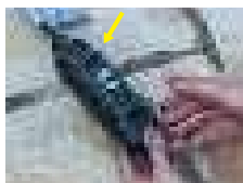
4. Press the «RESET» button, the indicator light turns red. The RCD works properly.
